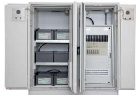
FZB Central Battery System in fire protection housing From page 27
