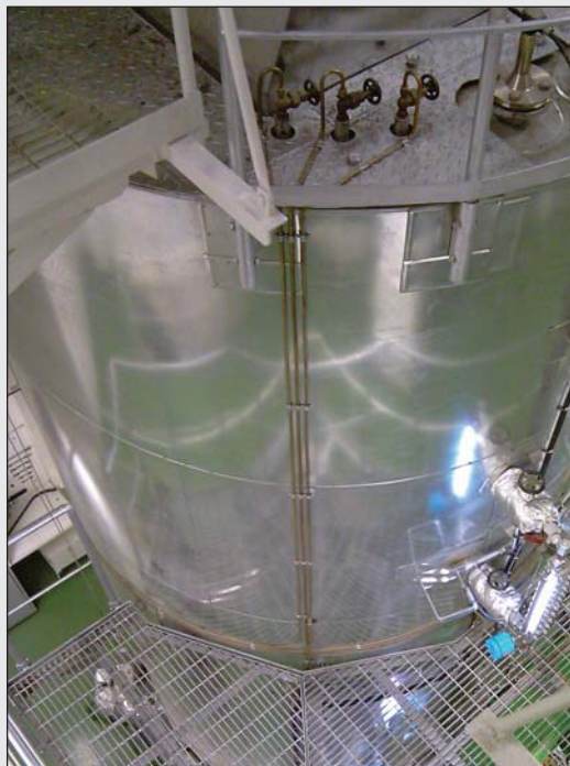
Marine Auxiliary Boiler
